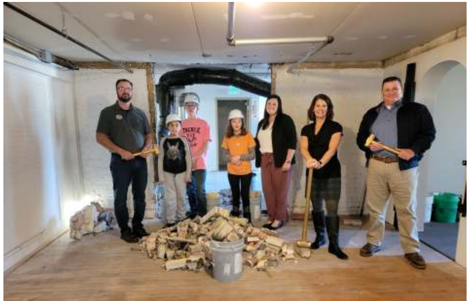
Formal kick off – “Groundbreaking” of the Community Center, 2802 Meadow Lane, Manitowoc, WI 54220. Renovation project of the upstairs for the purpose of further youth programming services. Pictured left to right: Dale Cayemberg, Ascend Services’ Director of Operations, youth clientele: Angel, Dominic, and Makenna; Marissa Fitzgerald, Ascend Services’ Program Director; Deanna Genske, Ascend’s Executive Director and Todd Wagner, Hamann Construction Project Manager.
